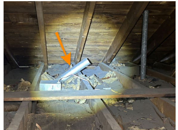
Bathroom exhaust vent
