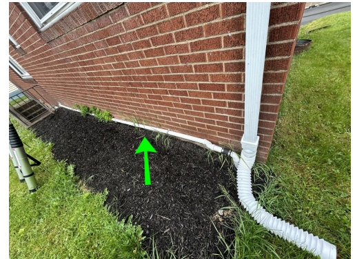
Sump Pump Discharge Pipe
